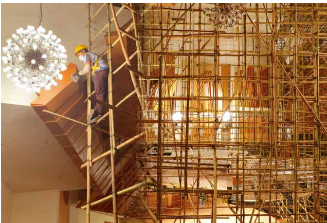
A six-storey scaffold was erected in the Concert Hall of the Hong Kong Cultural Centre so that cleaning of ceiling and acoustic panels could take place while the venue was closed due to COVID-19.
